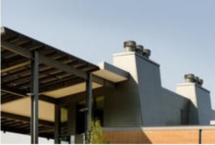
Ventilation stacks with wind-driven ventilation turbines. - Photo Credit: Stephen Miller
