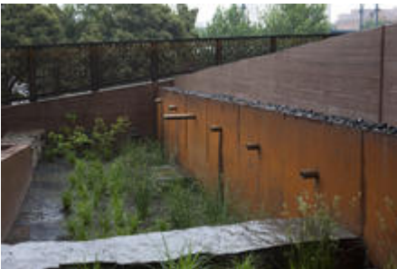
Another view of custom rainwater collection and stormwater treatment system. - Photo Credit: Sally Schoolmaster
